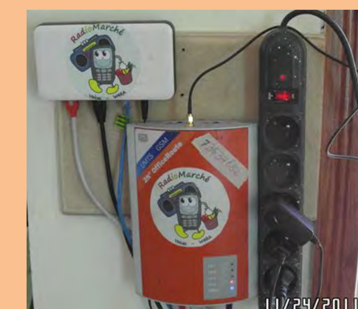
Locally deploy 2G phone hardware
